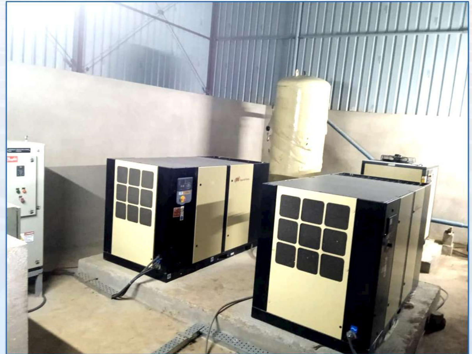
Air Compressor: Air compressors with collective capacity of 600 CFM at delivery of 8 PSI .
